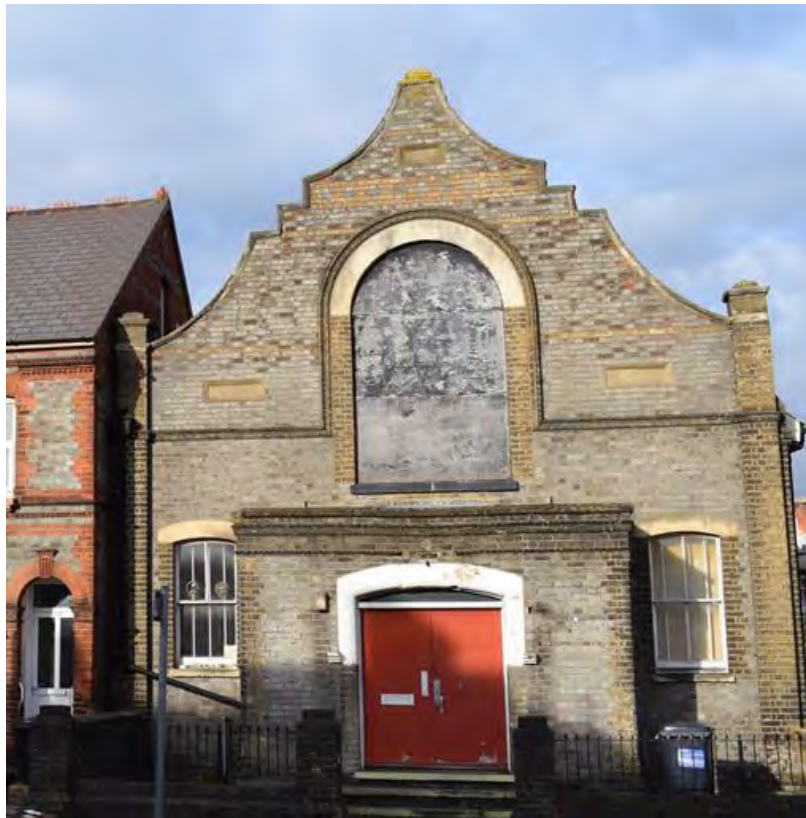
Figure 6.2.13 Bridge Hall, originally built for the Reading Open Brethren Group, in poor repair (David Neale)
