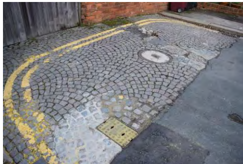
Figure 5.5.3 Sett stone pavement at the end of Belle Vue Road, still displaying the fan pattern of road that was common in the area (Karen Rowland)
