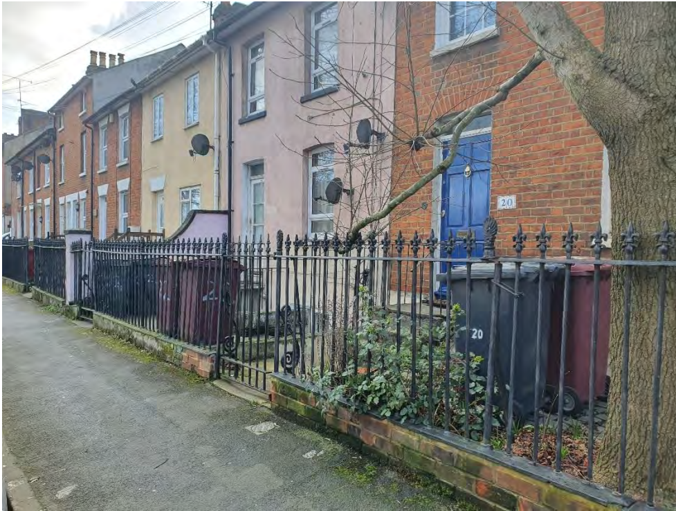
Figure 6.3.5 Original iron railings at 16-22 Howard Street and the curved stucco dividing wall at no. 22 (Mark Worringham)
