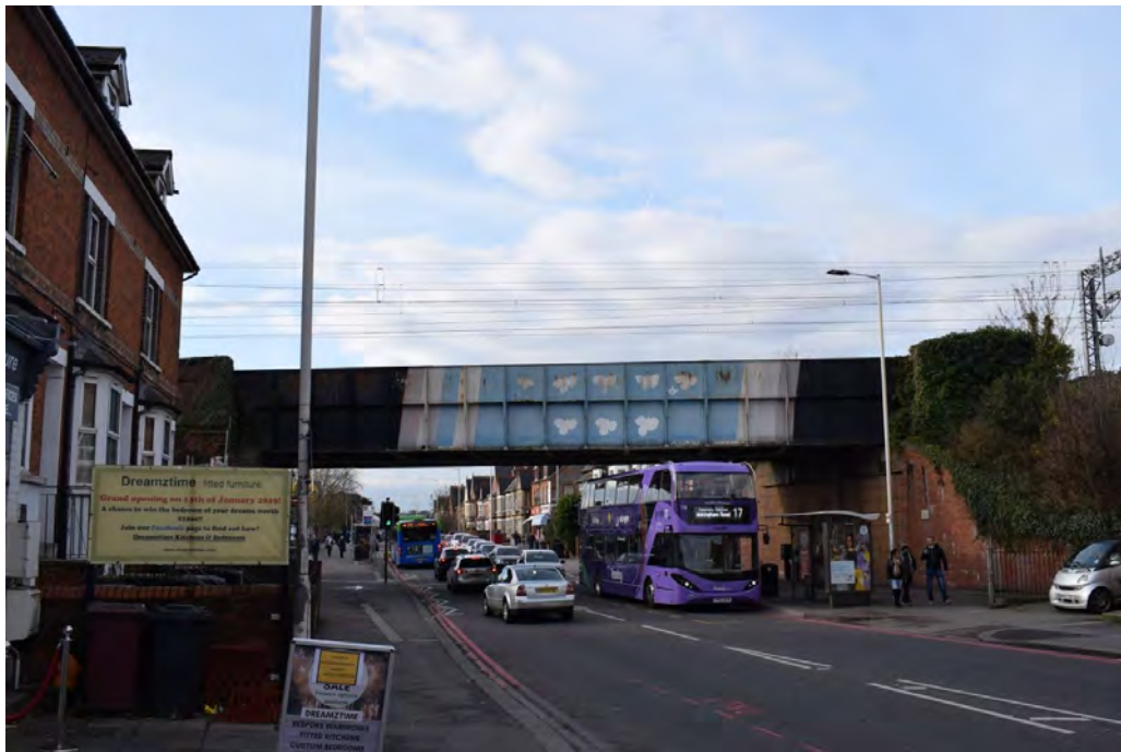
Figure 6.2.2 Reading West railway bridge, facing west along the Oxford Road, the iron bridge replaced an original brick design (David Neale)
